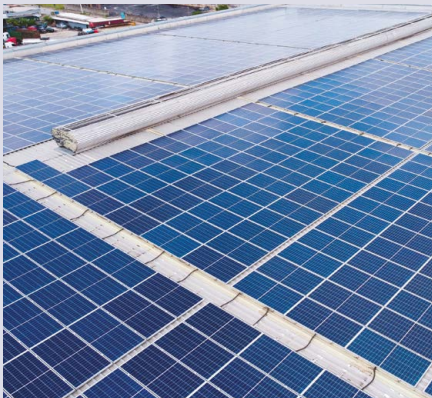
ROOF MOUNTED SYSTEMS
